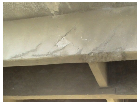
Crack in Gunited Girder
