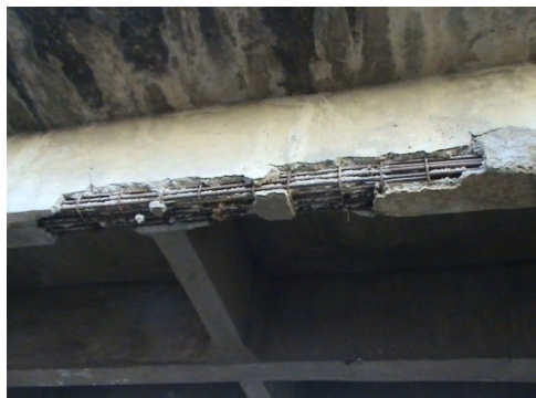
Damaged Girder - Before
